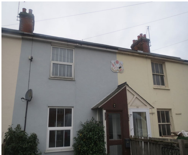
Figure 150 Visual comparison of historic retention of sash windows (right) and modern replacements (left)
