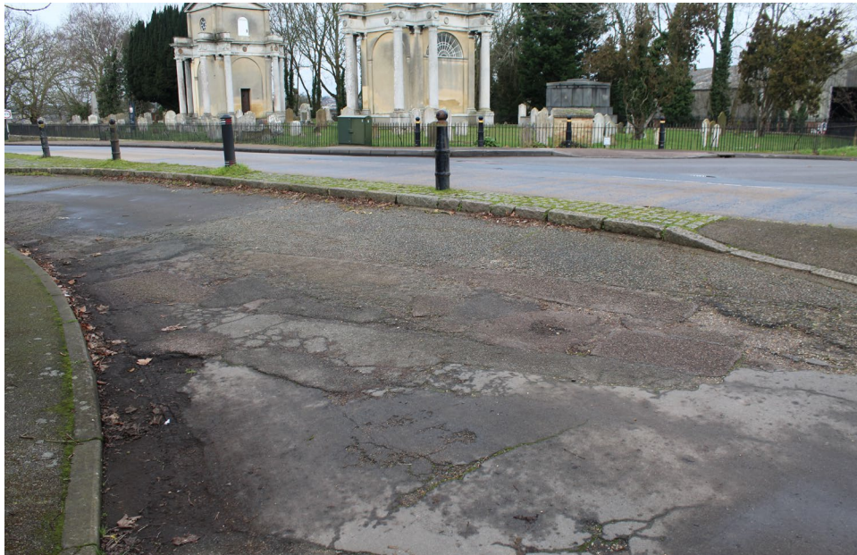
Figure 162 Poor surface treatments opposite Mistley Towers
